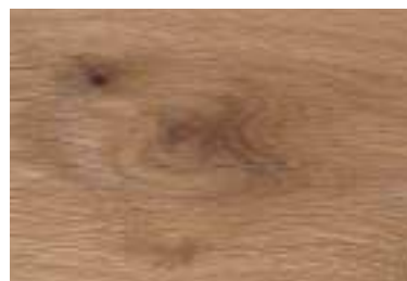
CHECK: A lengthwise opening on the face of the board resulting from rapid or faulty drying.
